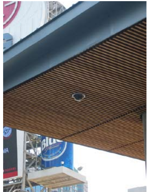
Security cameras keep a watchful eye on the activities within the square.
